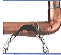
FROZEN PIPES & LEAKS
